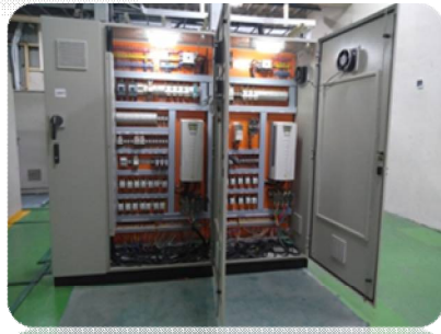
VFD Panel with Bypass & PLC
