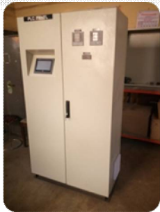
PLC Panel with 254 IO's
