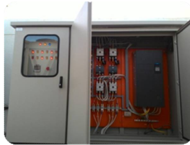
Chiller Compressor Panel
