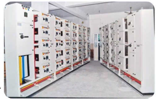
LT Panel for Power distribution and Motor Control up to 1000A
